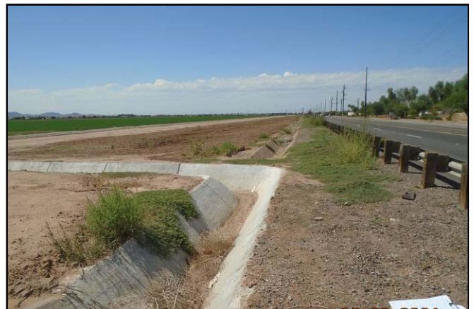
Picture 6 – MC85 / Buckeye Road, concrete irrigation canal near station 1208+00, right of centerline.
